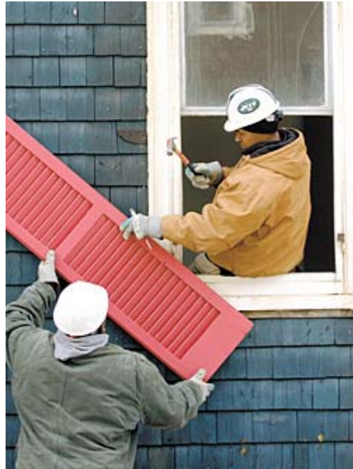
Lee Madison (left) and Dawnyah Smithson, employees of Baltimore-based Second Chance Inc., remove a shutter from a Towson office building before the structure is demolished.
